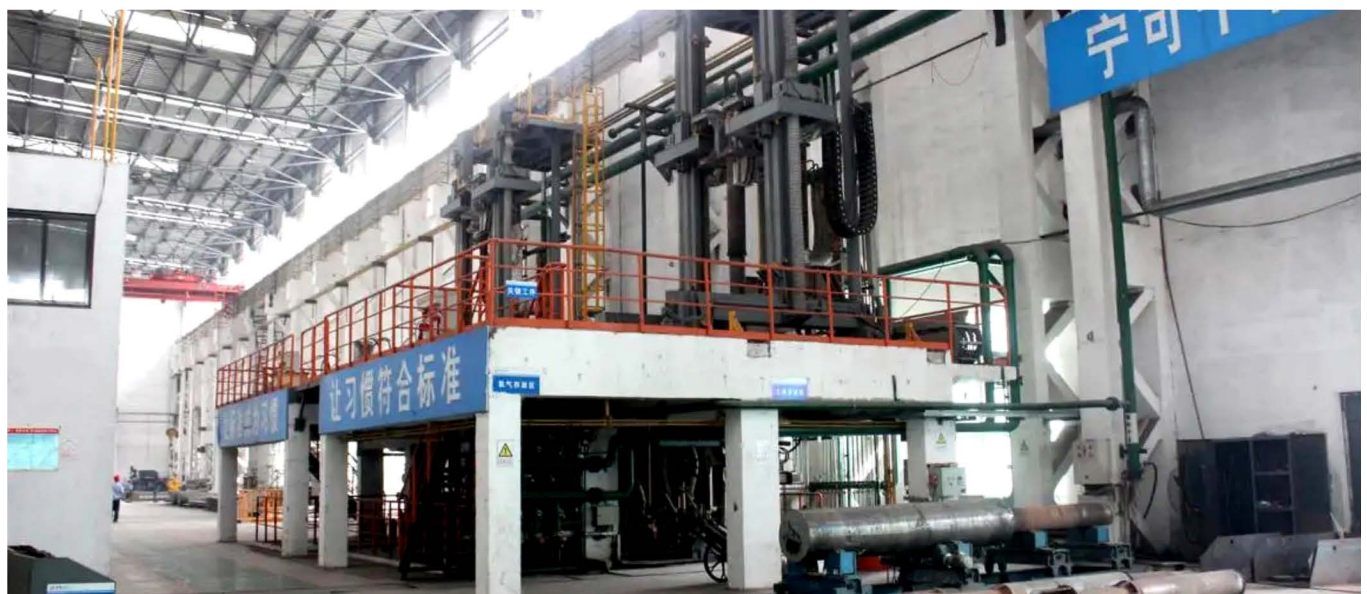
18 tons German ALD gas protection ingot electroslag furnace
