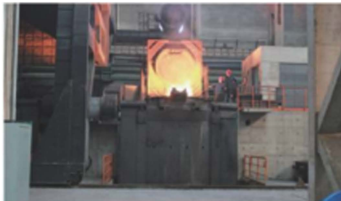
20-ton intermediate frequency induction furnace
